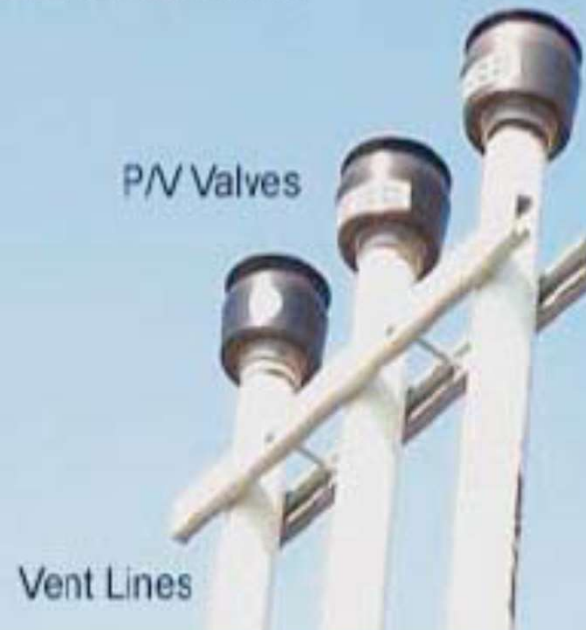
Three unmanifolded vent lines with three P/V Valves.
